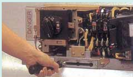
Releasing the mechanical lock at the disconnecting position by complete insertion of the lock collar
