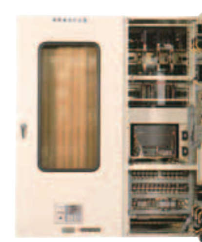
VCT盤 VCT panel
