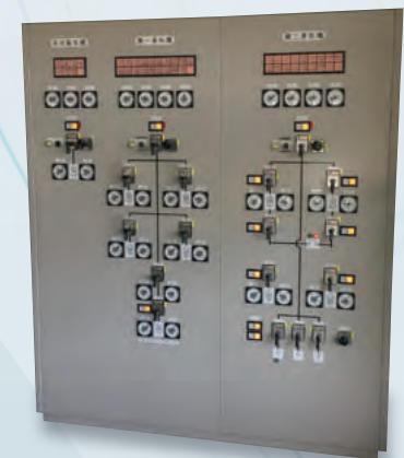
高圧電力監視盤 H/V & L/V DISTRIBUTION SUPERVISORY PANEL
