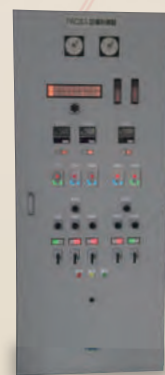
計装盤 INSTRUMENTATION PANEL
