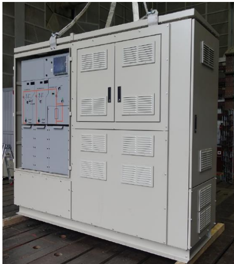
IAC-A (Door open condition)
