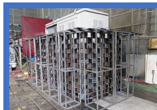
Indicators after the test Arc ignited in RMU
