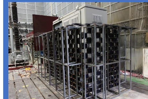
Indicators after the test Arc ignited in CC
